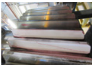
Crack inspection of the low-speed shaft gear wheel teeth
